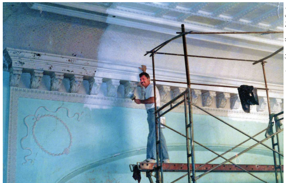
A worker paints the moulding in the Palaia Theater during its restoration.
